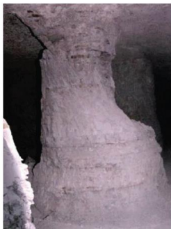
One of the irregular shaped and undersized pillars that failed during a recent mine collapse
