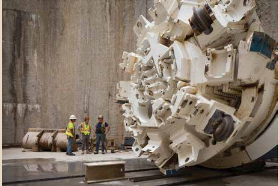
On April 30, 2015 in Honolulu, HI, a Robbins Main Beam TBM began a 4.6-km (2.8-mile) drive for a new sewer tunnel.
