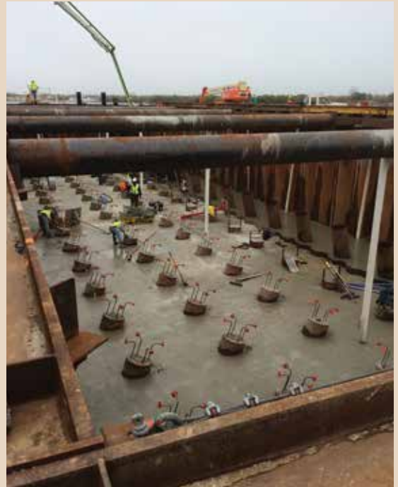
PCCP Project, a tour of the PCCP project was conducted in conjunction with RETC.
