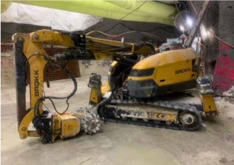
PCiRoads chose to partner with Brokk to rework more than 240 m (800 ft) of stormwater tunneling underneath the heart of Minneapolis.
