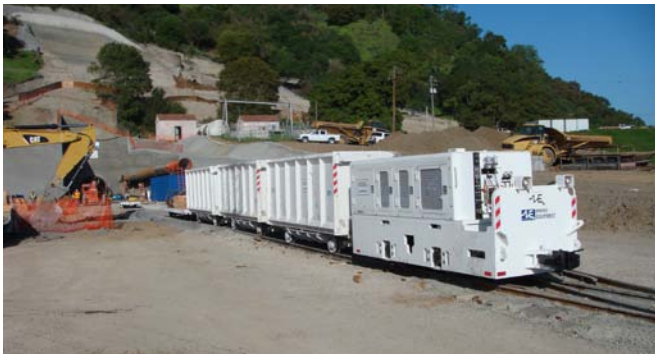
12-ton explosion proof diesel locomotive pulling 8 cubic meter side-dump muck cars out of the tunnel.
