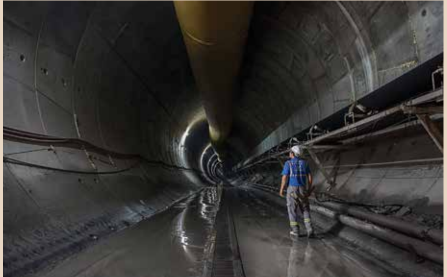
The Kargi Kizilirmak hydroelectric project, for Norwegian-owned Statkraft AS, will generate 470 GWh annually, which is enough to power about 150,000 homes.
