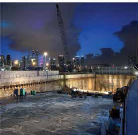
Above Left: Vargas Access Shaft New Irvington Tunnel, Fremont, CA. Left: Port of Miami Tunnel Miami, FL. Main: Bertha Rescue Shaft , Seattle, WA.
