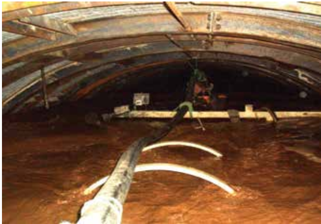
Parbati TBM buried in silt.
